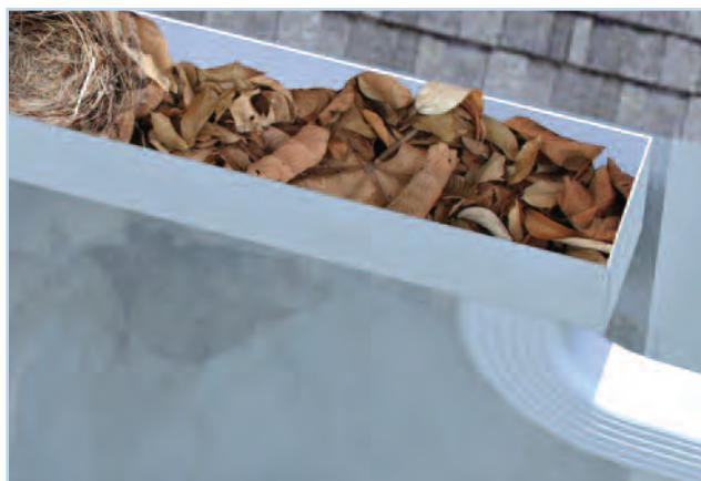
A clogged gutter can become a home for pests and prevents proper drainage away from the building.
